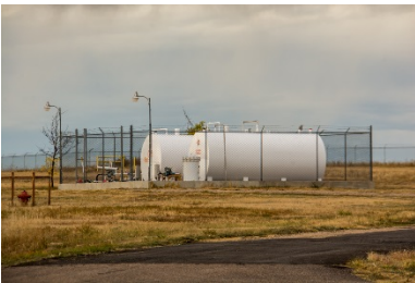
Aviation Fuel Farm & Containment Area
