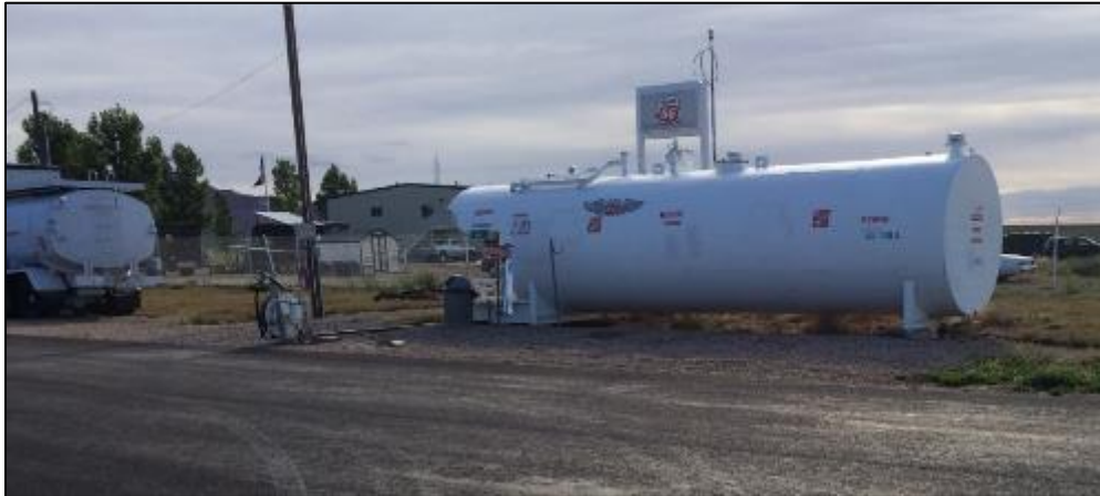
FIGURE 4-10 – 100LL AVGAS STORAGE TANK
