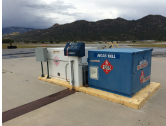
FIGURE 2-12 – SELF-SERVICE FUELING FACILITY
