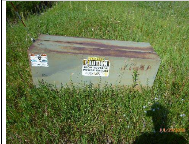
Electrical connection box along the south boundary of the subject property.
